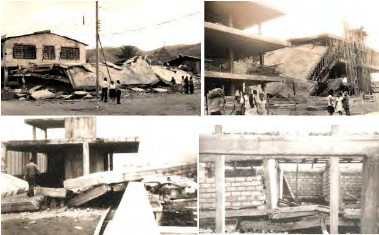
Figure 7a-d. Physical damage caused by the earthquake of 9 April 1976 (Mw 6.7). Upper images from left to right referred to the site of the school “5 de Agosto” and the Central Market. Lower images from left to right, referring to the damages of the “Delfina Torres de Concha” hospital and buildings of the company CEPE - Petroecuador, in the city of Esmeraldas. Photo courtesy: Triconsul.
