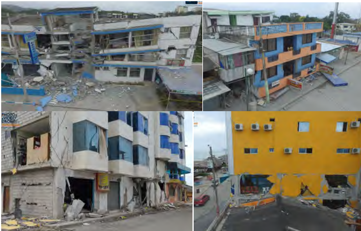
Figure 8a-d. Structural damage caused by the earthquake of 19 December 2016 (Mw 5.4, hypocenter 4 km). Upper images from left to right refer to the collapse of foundations at the Atacames site. Bottom images from left to right, referring to the site Tonsupa, province of Esmeraldas. Photo courtesy: "photo & video drone Esmeraldas".
