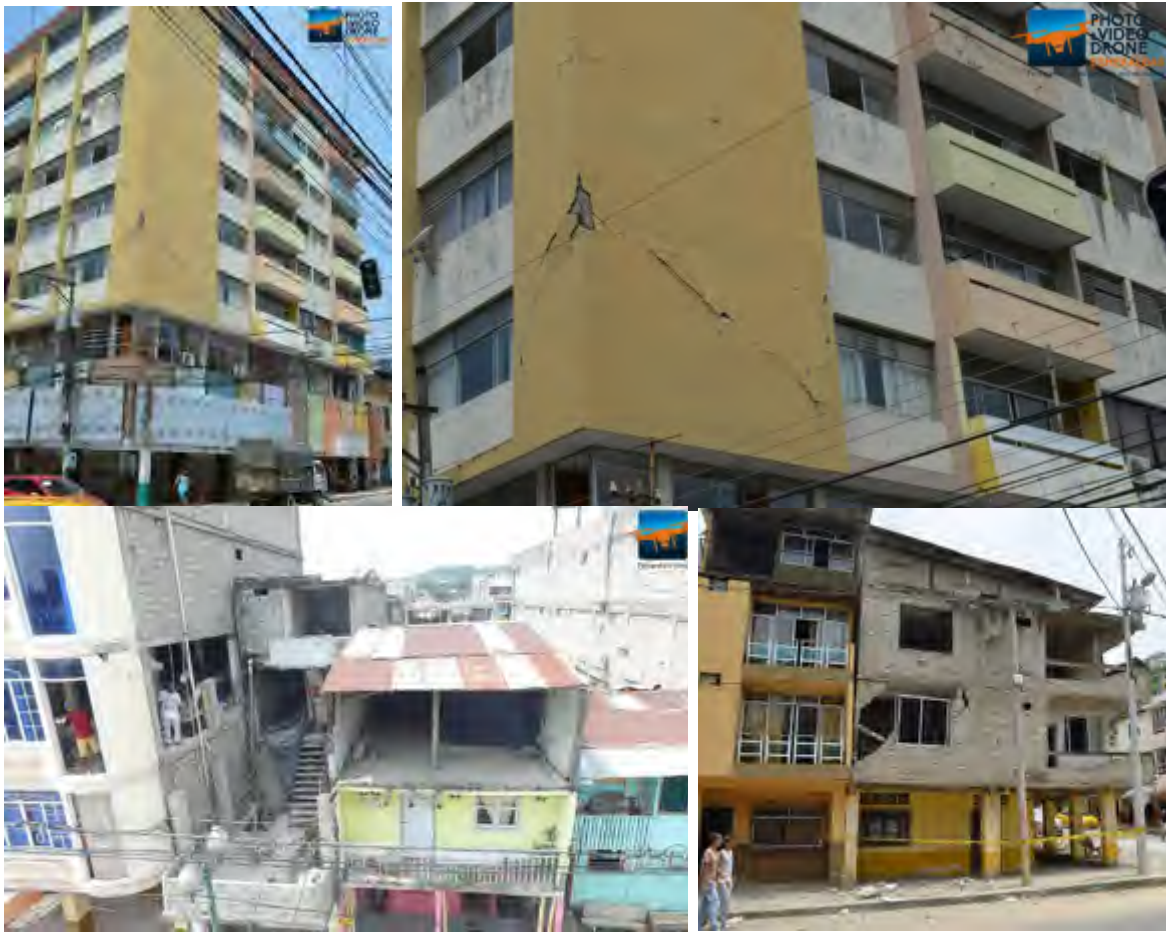
Figure 6a-d. Minor damage in the center of the city of Esmeraldas by the earthquake of Pedernales of April 16, 2016 (Mw 7.8). Upper images from left to right referring to the Bolivar and Manuela Cañizares direction. Bottom images from left to right, referring to the addresses December 6 and Piedrahita, and Ricaurte and / Colon and Eloy Alfaro. Photo courtesy: "photo & video drone Esmeraldas".
