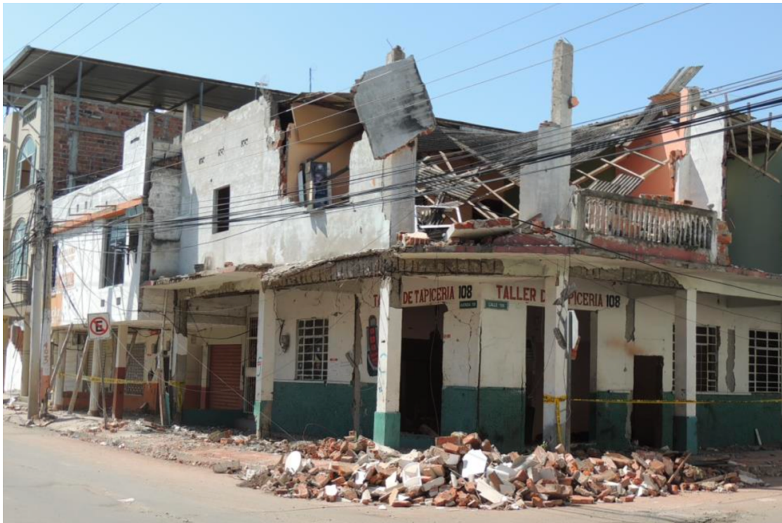
Fig. 7. Residential building in Tarqui, Manta, where the exterior walls collapsed. The roof also fell in this property. Adapted from Nicolaou et al. 2016.
