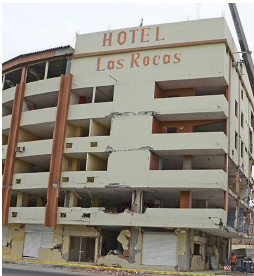
Fig. 8. This is how the building looked after the earthquake in Tarqui, due to the collapse of two floors it was decided to demolish it.
