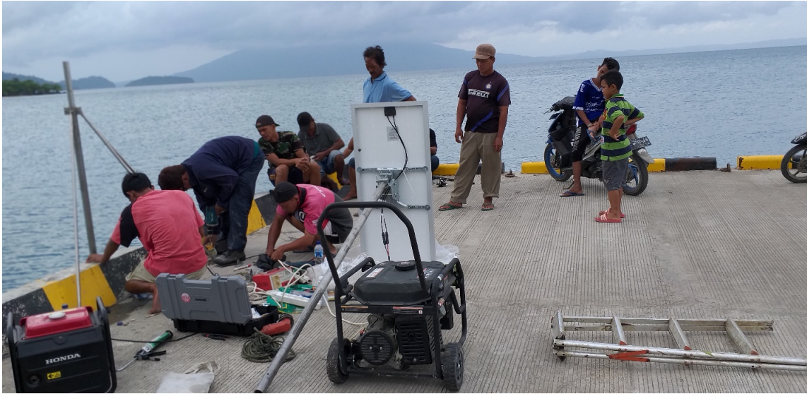
Figure 7 - The preparation of the installation of the IDSL in Sebesi island, followed by several local people
