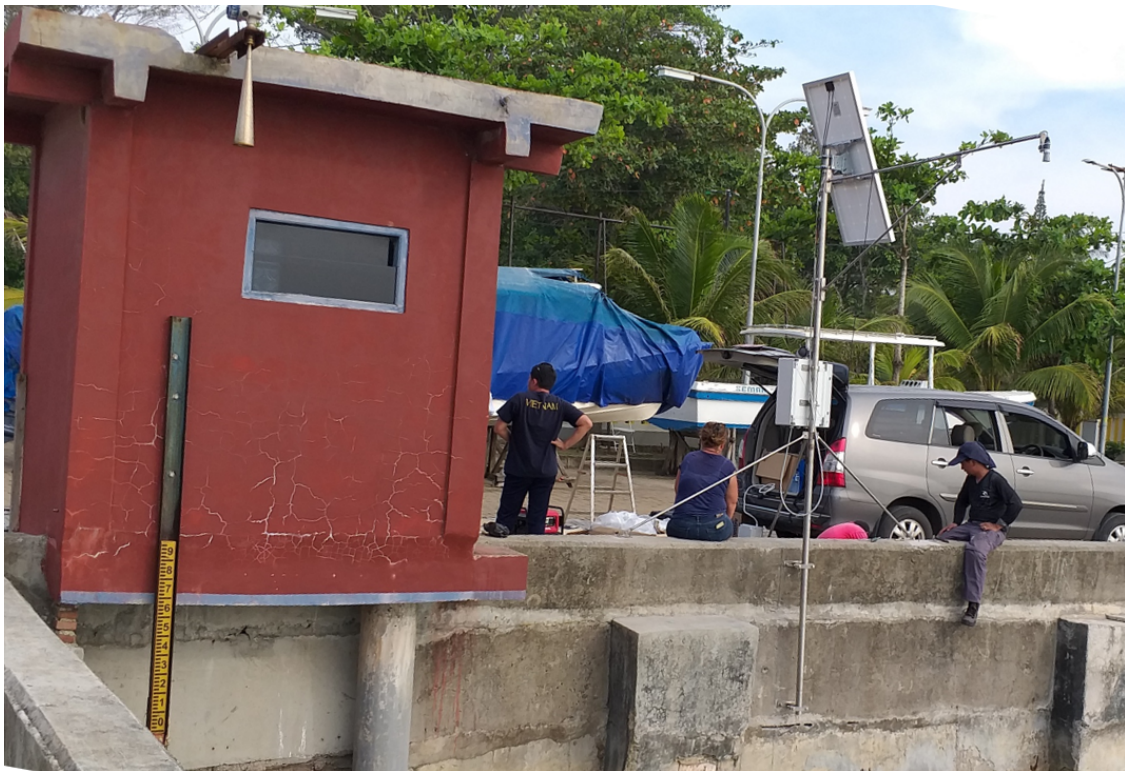
Figure 12 – On the left the BIG installation, on the right the IDSL device in Marina Jambu.
