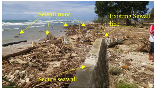
Figure 11. Seawall damaged at Batu Hideung Beach Banten
