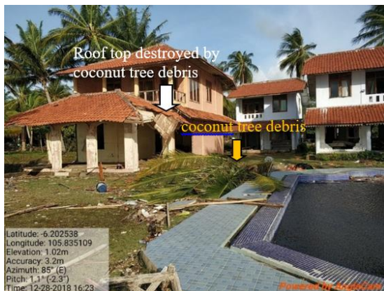
Figure 3. The rooftop of the building was damaged by a coconut tree debris
