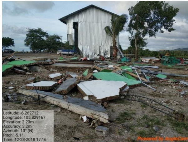
Figure 5. The damage warehouse (steel frame, thin sheet steel enclosure) and brick wall with reinforce concrete frame buildings
